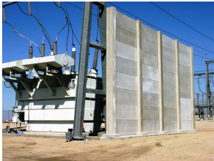
The installation is COMPLETE!
